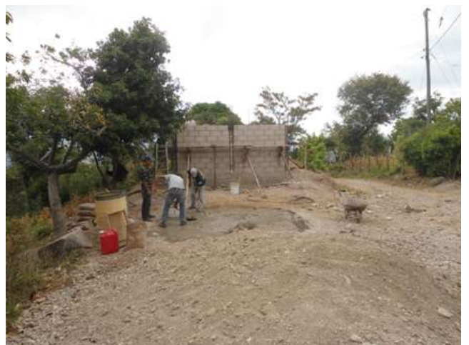
The distribution tank being constructed on a hill above the village to that the water to the homes of the residents will flow just with gravity.
